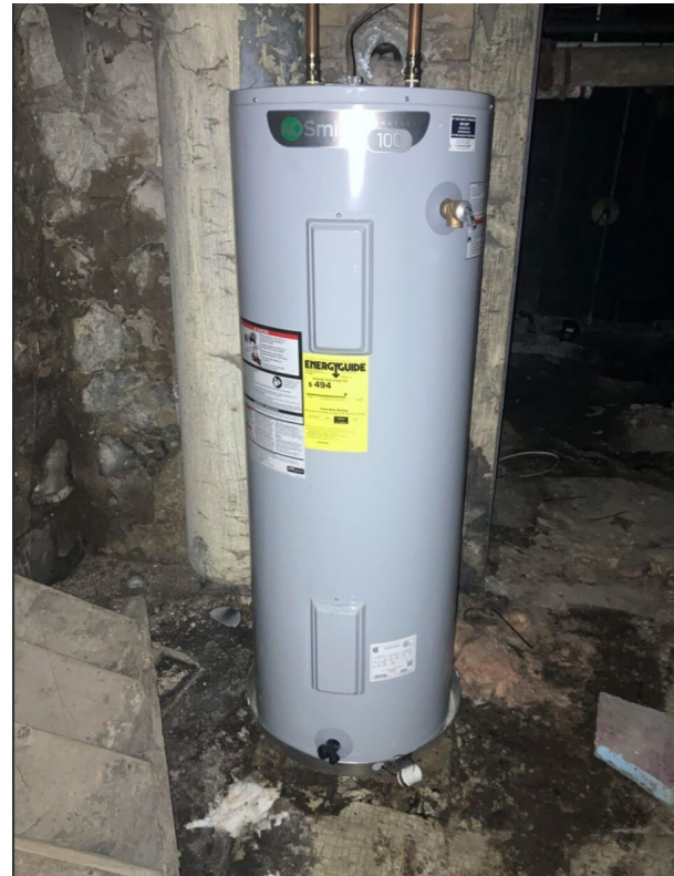
Water Heater After
